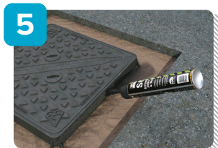
5 UltraCrete SCJ edge sealant and bitumen tack coat should be applied to all edges of the trim back and new frame.
