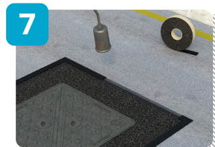
7 Once the surface course is compacted, apply UltraCrete Instaband ECO® thermoplastic overbanding to the edges of the reinstatement.
