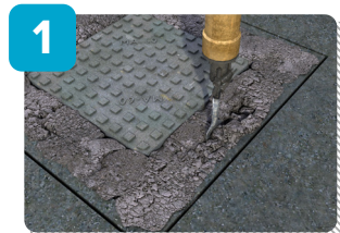
1 A picture frame is saw cut and excavated and the existing cover and frame removed.
